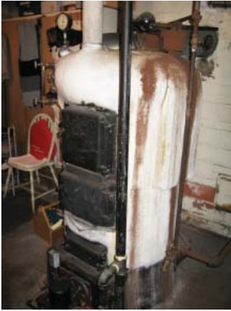
The Tamerlano's old furnace was covered with asbestos.
